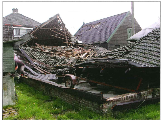
Figure 5. Damage of a (old) barn due to the tornado in Muiden on 23 August 2004 (photo by R. Sluijter).
