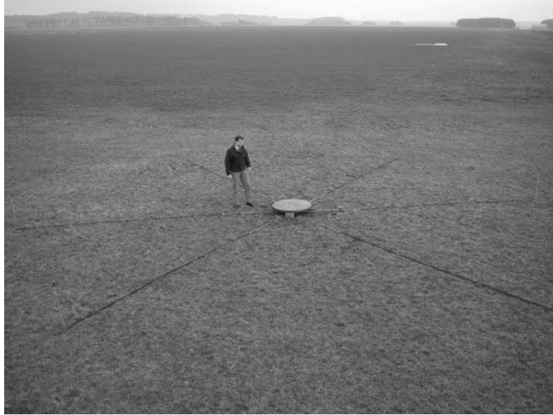
Figure 2.6: Installation of a microbarometer in DIA. The microbarometer is installed beneath the earth's surface and covered by a concrete top. The atmosphere is sampled by six porous hoses in a star-like layout, each of 5 m length.
